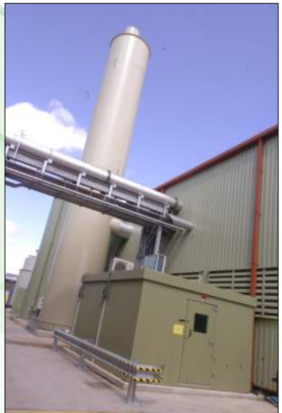
Flue Stack and ancillary equipment at the Dumfries Facility
